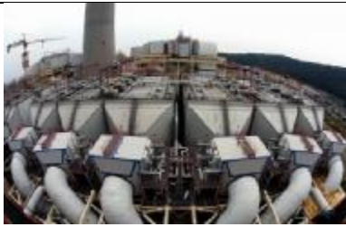
Figure 7. Operating ESPs of one 1000 MW coal-fired power unit in Zhejiang province
