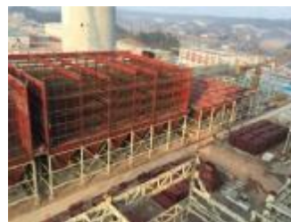
Figure 6. Installation ESPs of one 1000 MW coal-fired power unit in sichuan province
