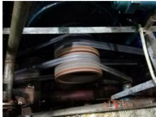
Figure 1. Failure state belt vibration amplitude
