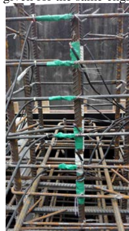
Figure 2. Seismic Performance of Reinforced Concrete Pier
