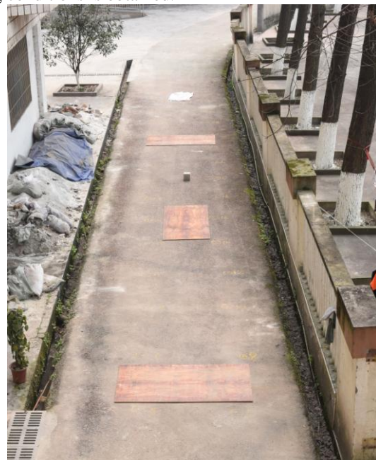
Figure 4. Local deformation condition of road
