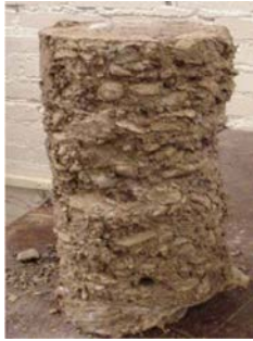
Figure 2. Material Degradation after Freeze-Thaw Cycles (Khoury 2005)
