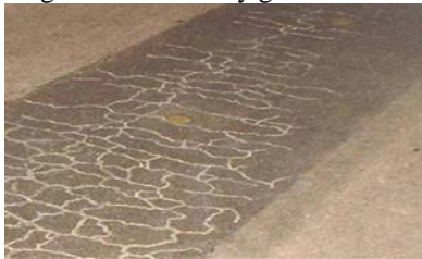
Figure 1. Fatigue Cracking in CSL (Yeo et al. 2002)
