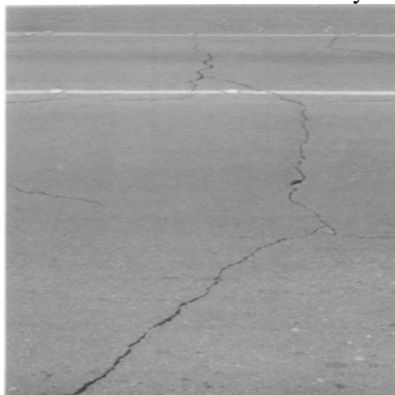
Figure 2. Transverse Cracking due to Shrinkage Cracking of CSL (Freeman and Little 2002)
