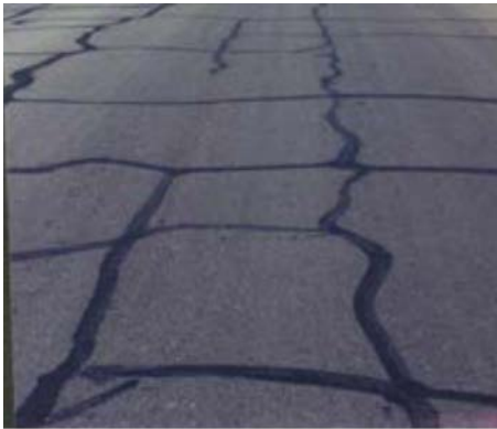
Figure 1. Block Cracking in HMA with Stabilized Base (Scullion 2002)
