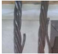
Figure 5. Destruction Form at Corrosion Rate of 8.72%
