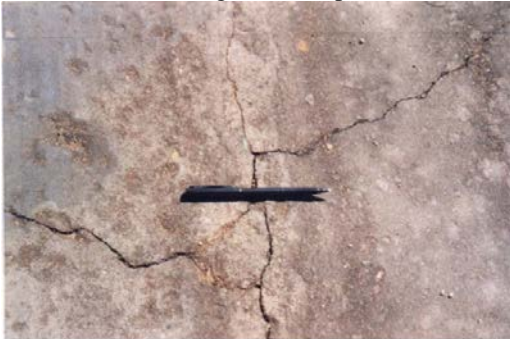
Figure 1. Shrinkage Cracking of CSL (George 2001)
