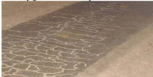
Figure 2. Fatigue Cracking in CSL (Yeo et al. 2002)
