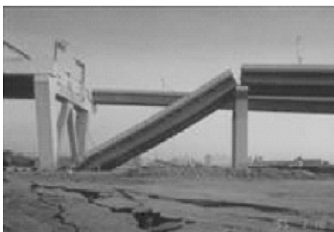
Figure 1 The falling beam of the approach bridge of Nishinomiya Bridge during the Kobe earthquake in Japan 图 1 日本神户地震中西宫桥引桥落梁破
