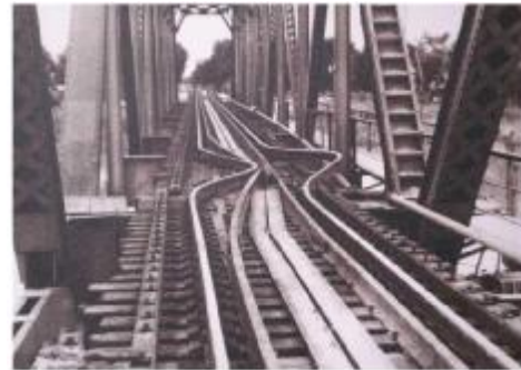
Figure 2 Torsion deformation of abutment of railway bridge during Tangshan earthquake 图 2 唐山地震中铁路桥的桥台扭转变形
