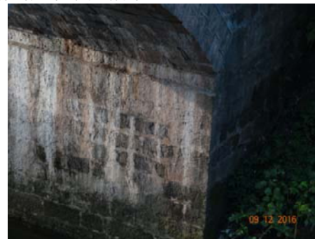
Figure 3. Weathering and Water Erosion of Arch Bridges 图 3. 拱桥的风化、流水侵蚀
