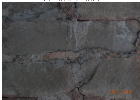
Figure 2. Vault Longitudinal Cra 图 2. 拱顶纵向裂缝
