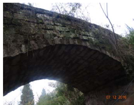
Figure 4. Ash Joints of Arch Bridge Fall off 图 4. 拱桥的灰缝脱落
